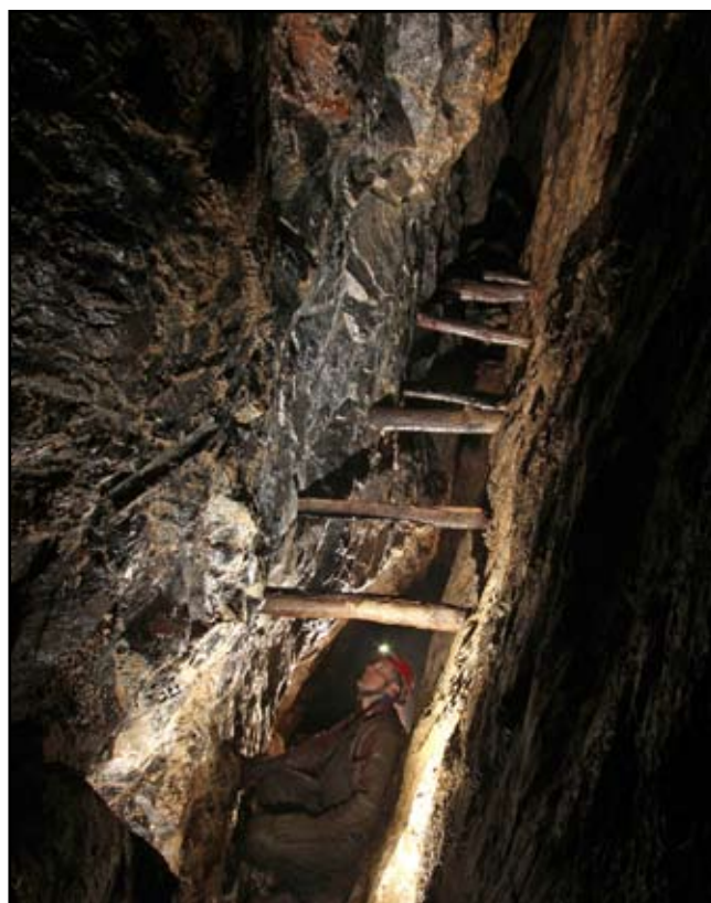
Figure 20. A line of stemples across a slope in "old man" workings in a higher part of the vein (photo: Rob Eavis).
